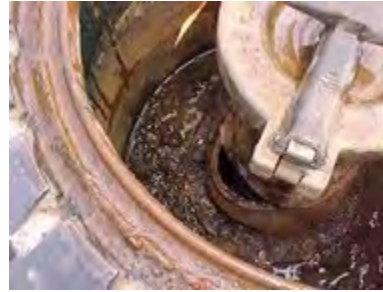
Figure 18. Image of spill bucket.
