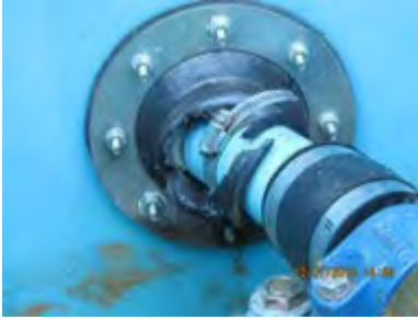
Figure 17. Image of sump boot.
