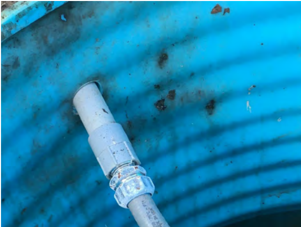
Figure 19. Image of unsealed penetration in containment and residue present.
