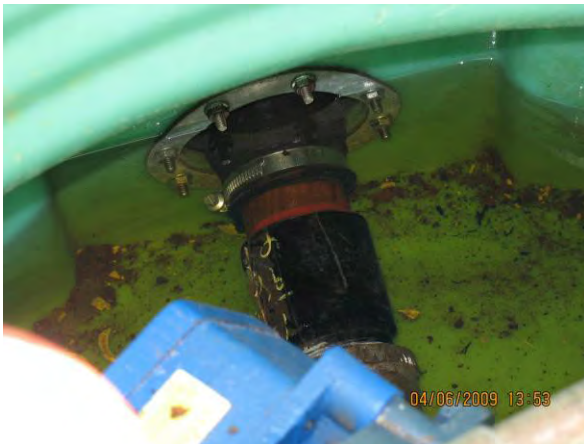
Figure 21. Failed entry boots leading to water in the sump.
