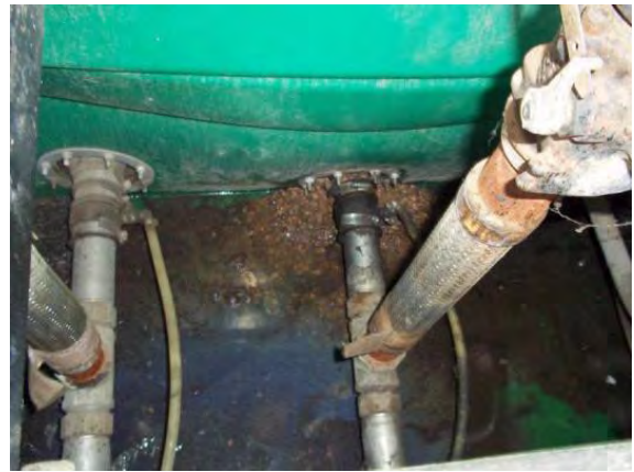
Figure 24. Compromised sump indicating the sump is not “water tight.”
