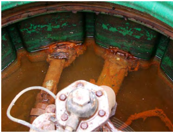
Figure 23. Water in the sump, integrity (find buckling along wall of sump).
