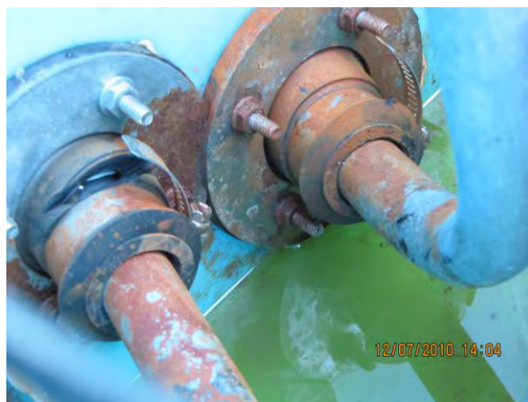
Figure 22. Failed entry boots allowing water into the sump.
